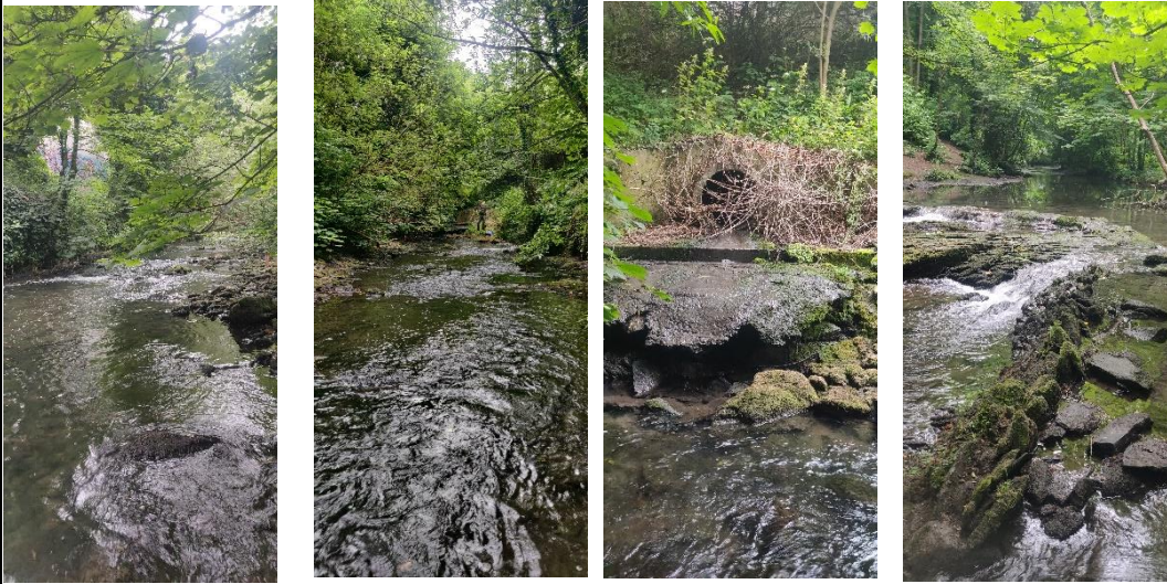
From left to right: the survey location looking upstream, the survey location looking downstream, the culvert pipe located on the right bank, the waterfall/bedrock outcrop upstream of the survey location.
